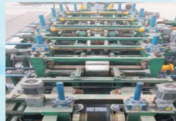
325mm ERW Pipe Mill
