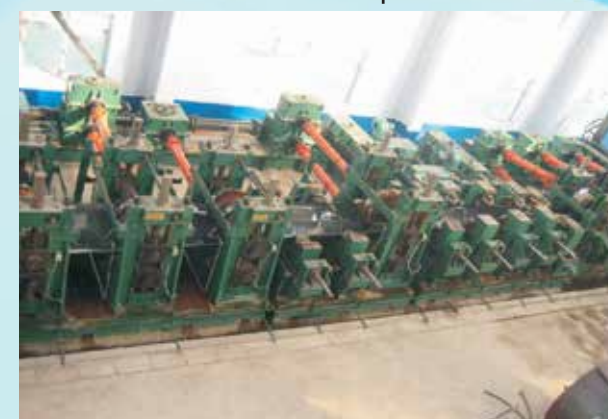
406mm ERW Pipe Mill
